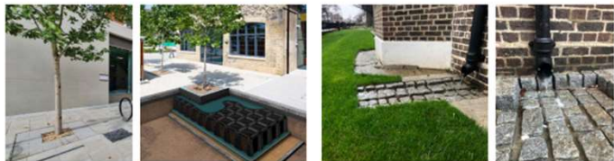
⑤ Engineered tree pits that manage rain water run off and benefit longterm tree health.
