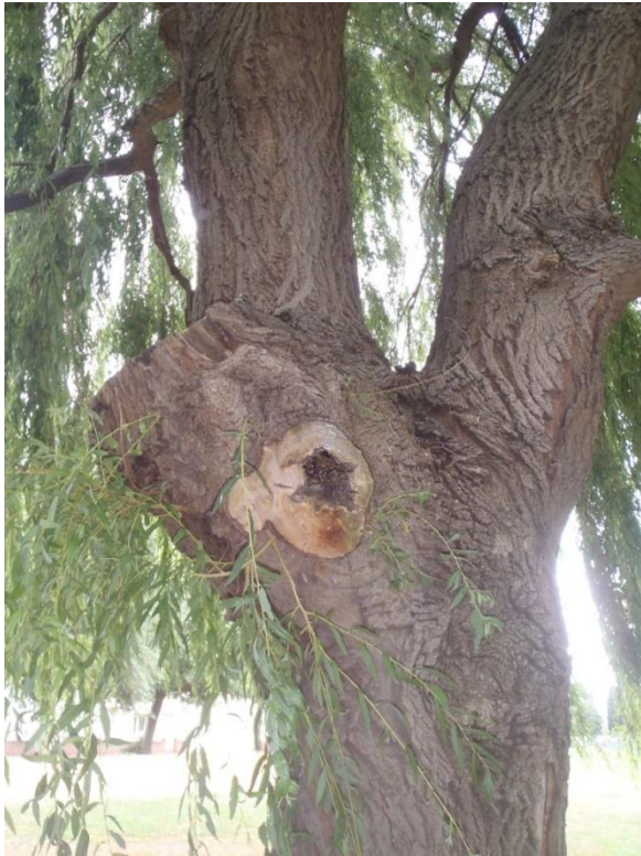
Photograph 9 –View of tree (1) with potential bat roost located on the amenity grassland (refer to Figure 2)
