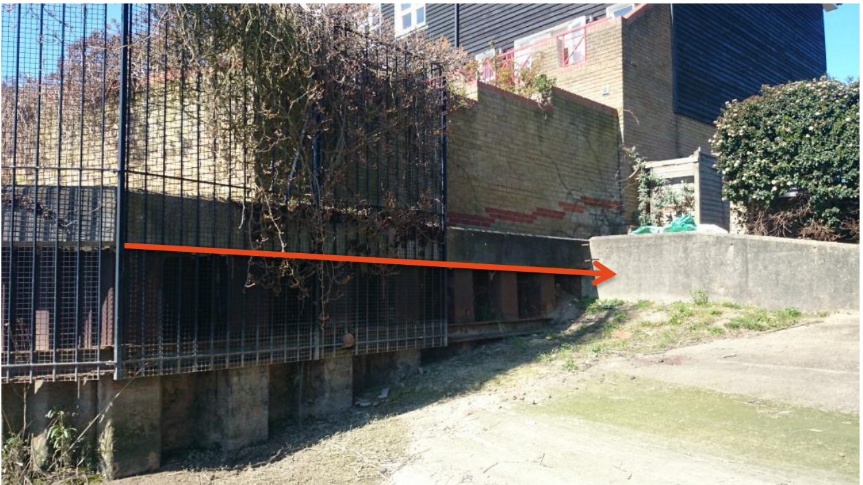
Photograph 4 – Showing point H - A cantilever type addition would be required to allow the passage of walkers across the slipway (see red arrow).
